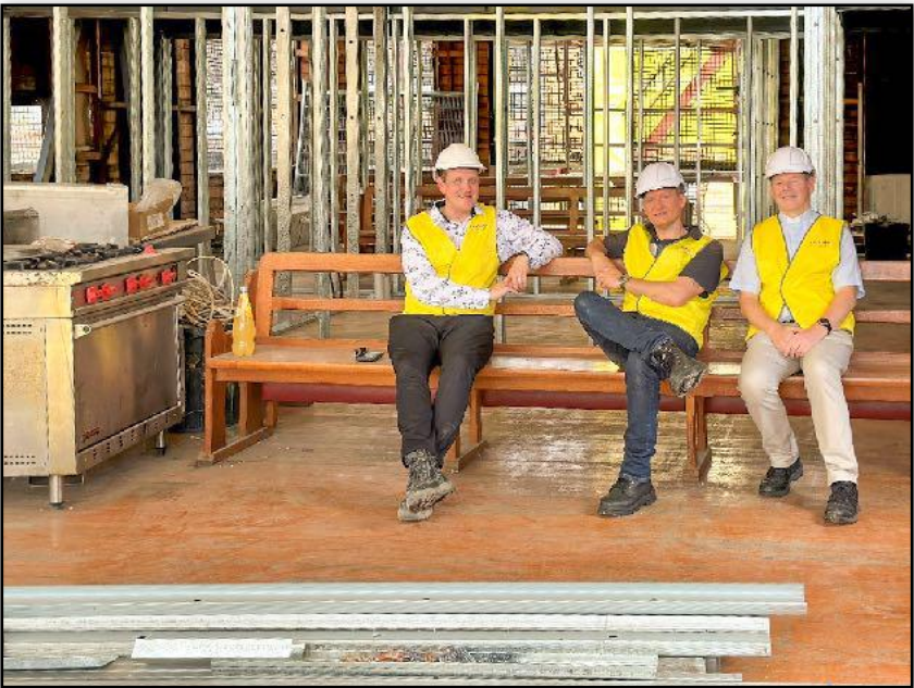
Inside the old hall, the framing for the new rooms has commenced
