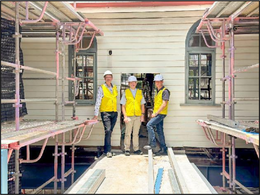
The new bridge link between the new hall and the old hall
