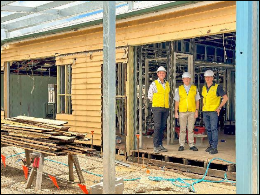
The rear of the old house, being remodelled as part of the ELC
